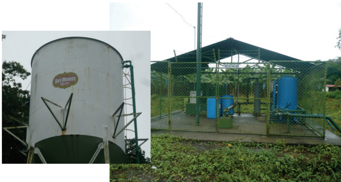
Figure 7. Water tank and well for drinking-water extraction in Bananita.
